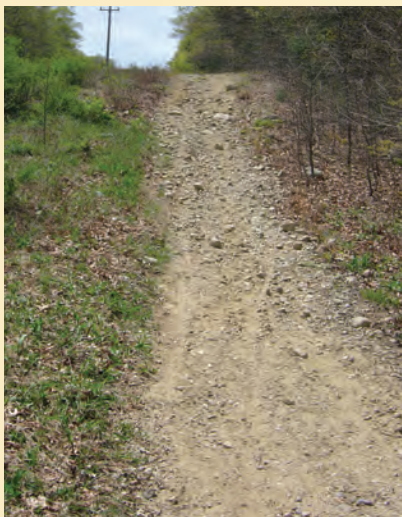
The east side of CHR under the utility lines would benefit greatly from a series of waterbars.
