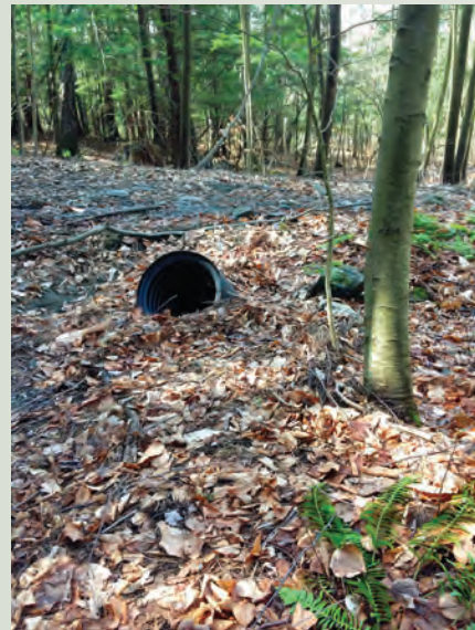
This culvert collapsed from an extreme rain event, initiating a major erosion problem.
