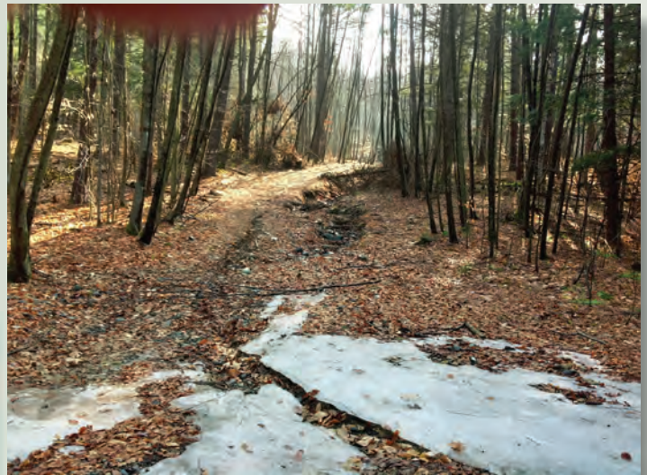
The fire road's straight, steep slope makes it vulnerable to heavy erosion. Today it is impassable.
