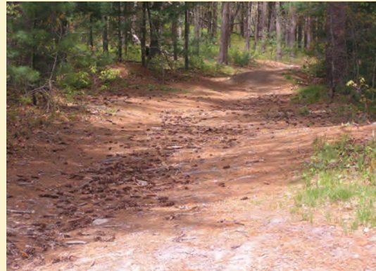
Excessive widening increases rapid runoff and sedimentation of waterways.
